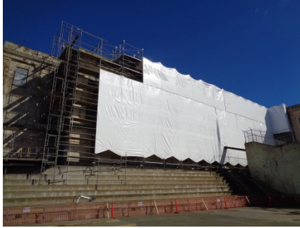
Shrink wrapping provides a visual barrier so that work does not disturb the island's birds.
